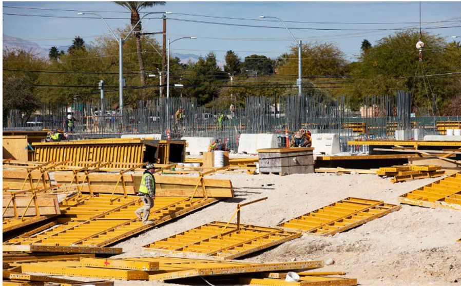
Construction workers work on the future medical education building for UNLV's School of Medicine in Las Vegas, Wednesday, Jan. 20, 2021. (Rachel Aston/Las Vegas Review-Journal) @rookie__rae
