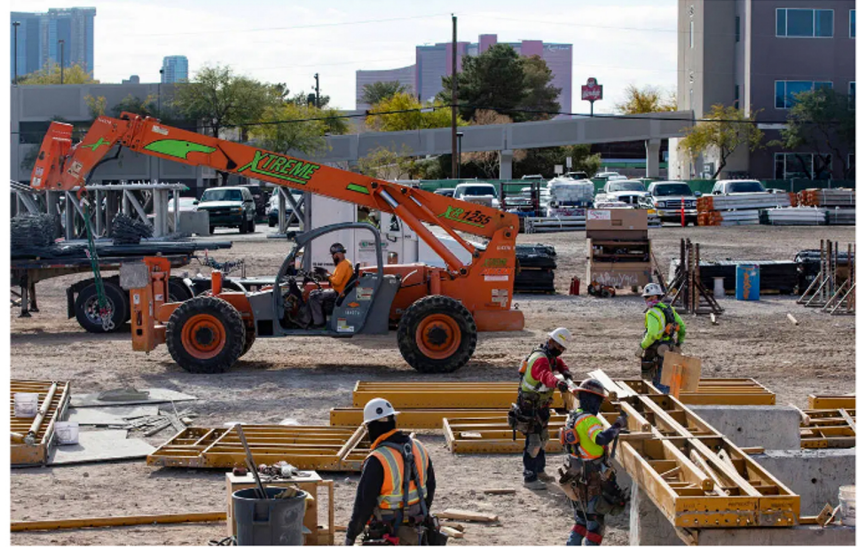
Construction workers work on the future medical education building for UNLV's School of Medicine in Las Vegas, Wednesday, Jan. 20, 2021. (Rachel Aston/Las Vegas Review-Journal) @rookie__rae
