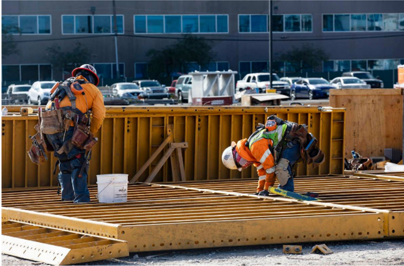
Construction workers work on the future medical education building for UNLV's School of Medicine in Las Vegas, Wednesday, Jan. 20, 2021. (Rachel Aston/Las Vegas Review-Journal) @rookie__rae
