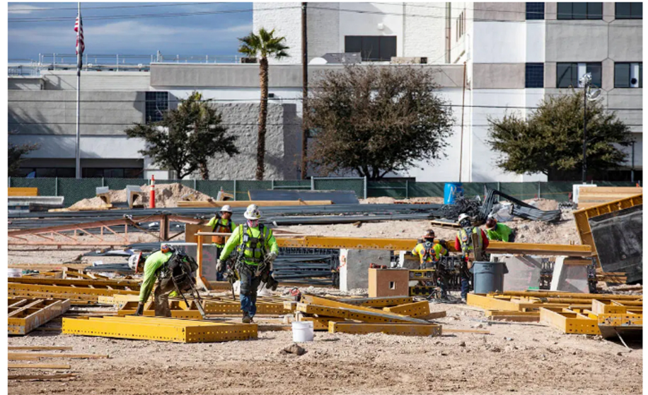
Construction workers work on the future medical education building for UNLV's School of Medicine in Las Vegas, Wednesday, Jan. 20, 2021. (Rachel Aston/Las Vegas Review-Journal) @rookie__rae
