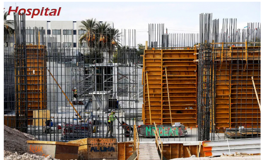
Construction workers work on the future medical education building for UNLV's School of Medicine in Las Vegas, Wednesday, Jan. 20, 2021. (Rachel Aston/Las Vegas Review-Journal) @rookie__rae
