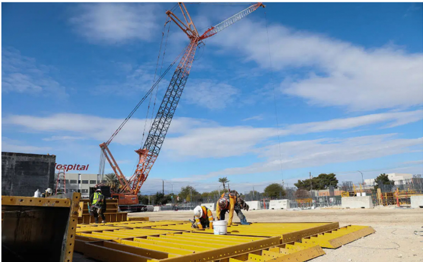
Construction workers work on the future medical education building for UNLV's School of Medicine in Las Vegas, Wednesday, Jan. 20, 2021. (Rachel Aston/Las Vegas Review-Journal) @rookie__rae
